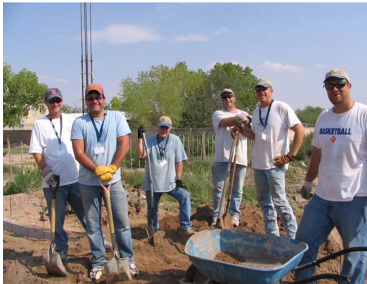
Guy Wade, Randy Ismond, Noel Kohler, Joel Zeller, Todd Graham and Lane Seaman working on the foundation.
